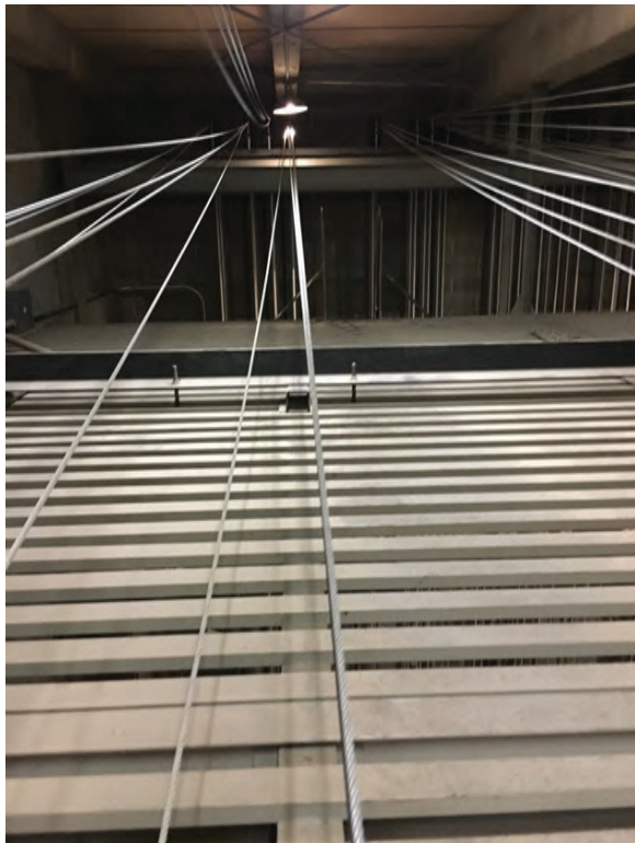
The image above shows unacceptable fleet angles coming off the headblock to the loft block.
