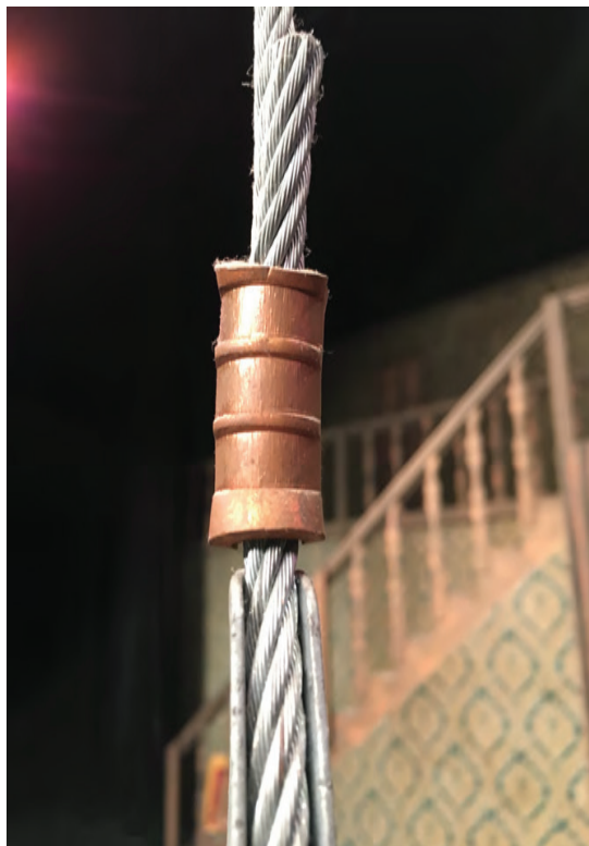
The picture above is appropriately terminated. (picture from another theater)
