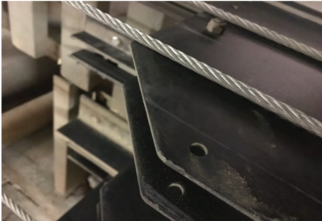
Picture above shows where cable is rubbing against the cheek of the loft block.
