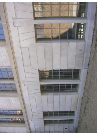
Figure 90. Care was taken to replicate the characteristics of the historic windows in these replacement units installed as part of the rehabilitation of the Chemistry Building.
