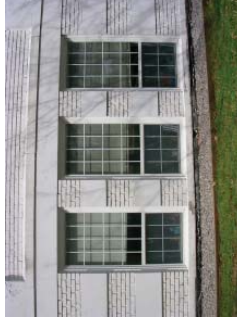
Figure 89. The replacement window units installed at Peabody Hall are comprised of single panes of glass with applied muntins. This approach does not capture the subtle characteristics of the original windows.
