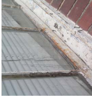
Figure 88. Close-up view of deteriorated steel window at Phi Delta Theta fraternity house.
