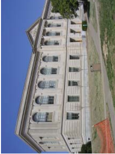
Figure 87. The windows of Vol Walker Hall are important character-defining features of the building and should be preserved.
