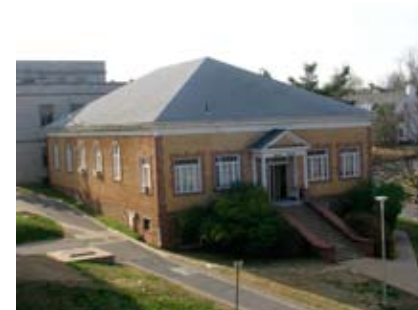
Figure 80. The Roof Condition Database indicates the roof of the Army ROTC Building is overdue for replacement.
