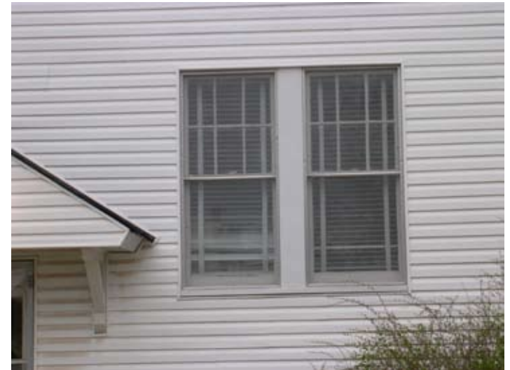
Figure 109. The application of the imitative siding has obscured the building's architectural detail and diminished its historic character.
