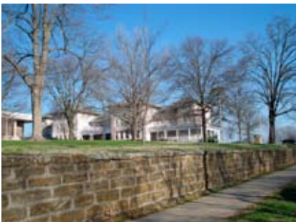
Figure 123. The stone retaining wall that defines the perimeter of Old Main lawn is an important landscape element that should be preserved and maintained.
