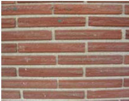
Figure 94. View of roman bricks used in the construction of the Phoenix House.
