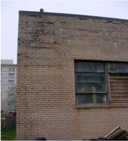
Figure 122. As the University's buildings age, repair and maintenance of historic materials will become increasingly important.
