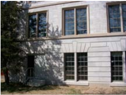
Figure 82. Proximity of trees to historic masonry can trap moisture and contribute to deterioration of the building envelope.
