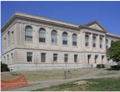
Figure 87. The windows of Vol Walker Hall are important character-defining features of the building and should be preserved.
