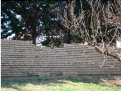
Figure 81. The retaining wall surrounding the Fine Arts Center outdoor amphitheater is in critical condition.
