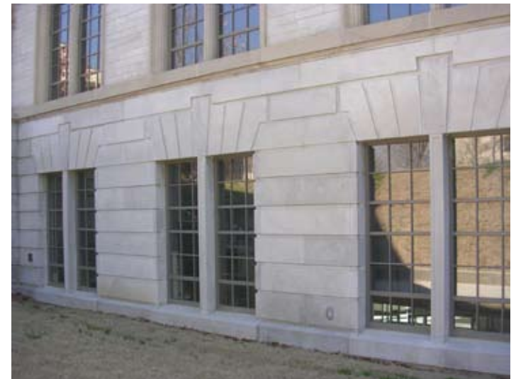
Figure 90. Care was taken to replicate the characteristics of the historic windows in these replacement units installed as part of the rehabilitation of the Chemistry Building.
