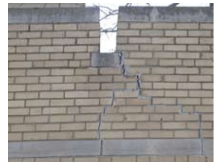
Figure 98. The Geology Building is suffering from severe masonry problems due to differential settlement.
