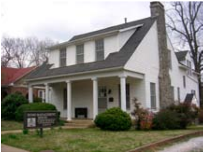
Figure 107. The replacement of the original porch columns and installation of imitative siding have diminished the character of this building.
