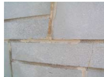
Figure 78. Close-up view of masonry joint repair made with non-matching mortar.
