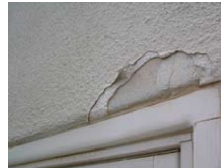
Figure 97. Some minor bubbling is occurring behind the painted coating recently applied over the stucco exterior of the Chi Omega Greek Theatre.
