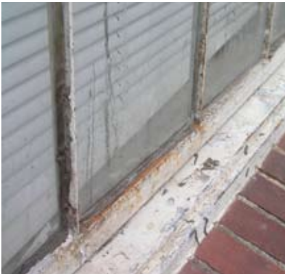
Figure 88. Close-up view of deteriorated steel window at Phi Delta Theta fraternity house.
