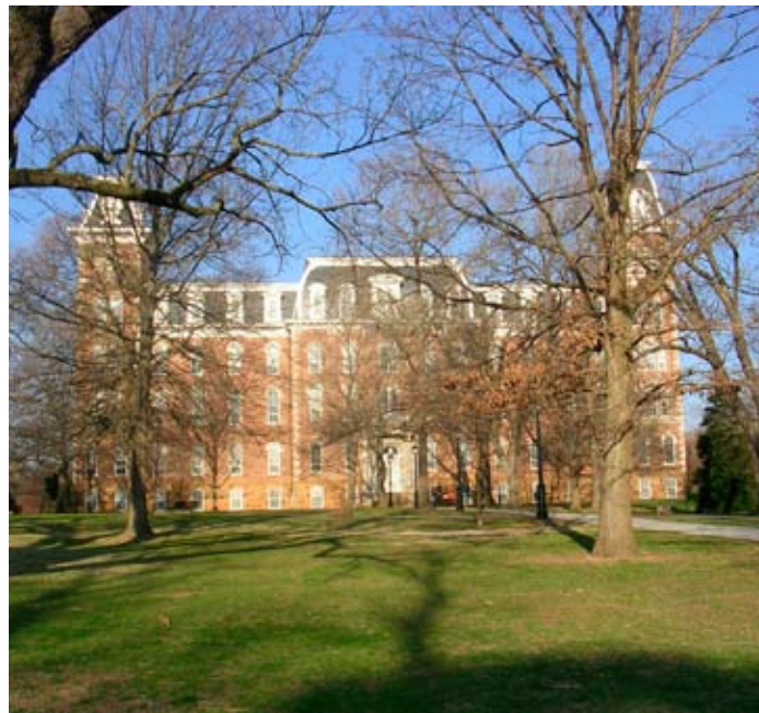
Figure 46. View of south tower of Old Main while under construction during the 1991 rehabilitation.
