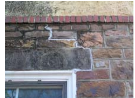
Figure 96. Sealant has been used to repoint this settlement crack in the base of the Army ROTC Building.
