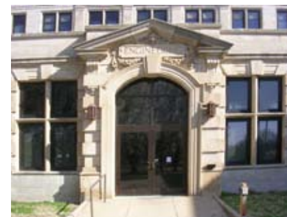
Figure 79. Replacement of original window and doors with bronze aluminum units has diminished the historic character of this building. Also note the replacement light fixtures flanking the entrance.
