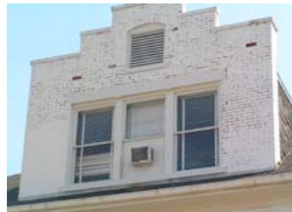
Figure 95. The parapet wall of the Agriculture Annex is suffering from joint deterioration and spalling of the host masonry.
